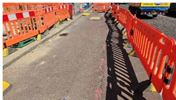
Fig 4.2: poor and rough paving in bus lane
