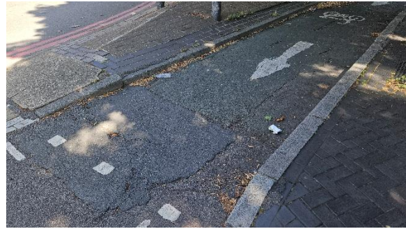
Fig 13.2: very poor surfacing on bypass
